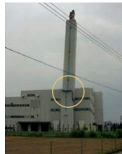
Stack which was broken at a height of about 18 m above the ground (near the top of the building) (just after the earthquake)
