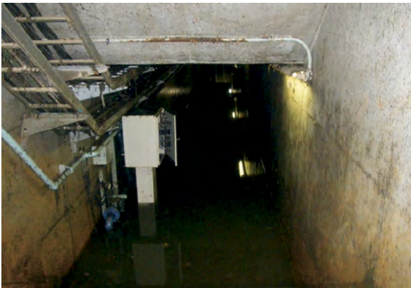
2 nd water treatment piping gallery
