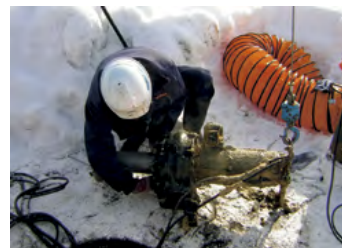
An example of maintenance work (responding to failure of a submersible pump in the snow)
