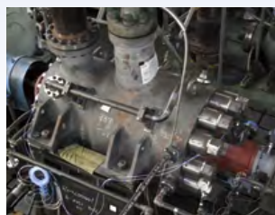
Boiler water supply pump for electric power plant
