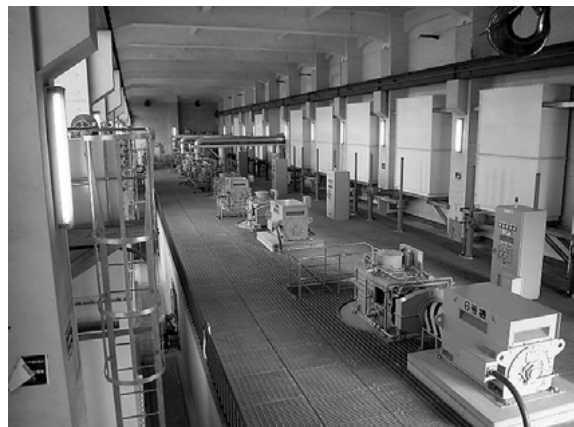
改修後ポンプ室内全景 Driver room after renovation
